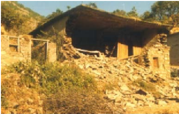
Partial collapse of non engineered building (stone masonry walls) during 1991 Uttarkashi earthquake. (Source: Earthquake Tips IITK-BMTPC)
