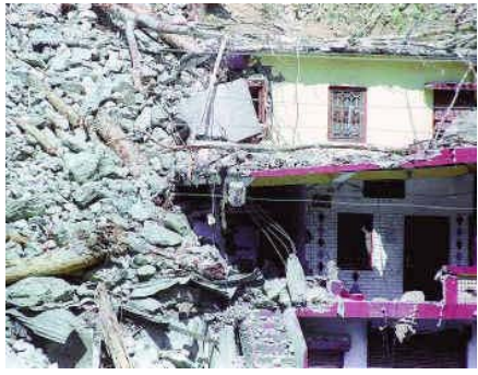
(Bottom Left): The Varunavat mountain rising on the edge of Uttarkashi town. Huge cracks on its side have set off several landslides. A building in danger of being buried. (Bottom Right): A building partly buried under rocks and other debris.
