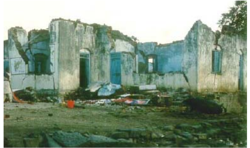
(a) Building with no horizontal lintel band: collapse of roof and walls
