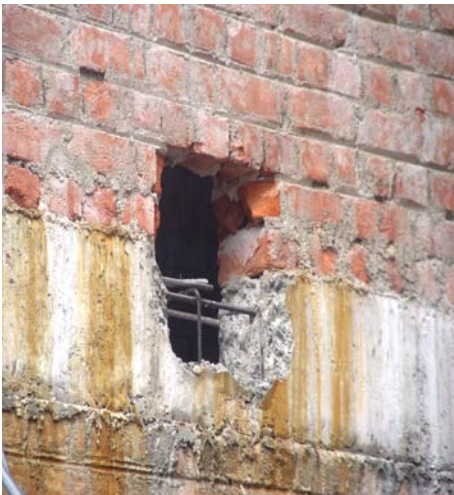
Figure 9.12: Disturbance of structural elements
