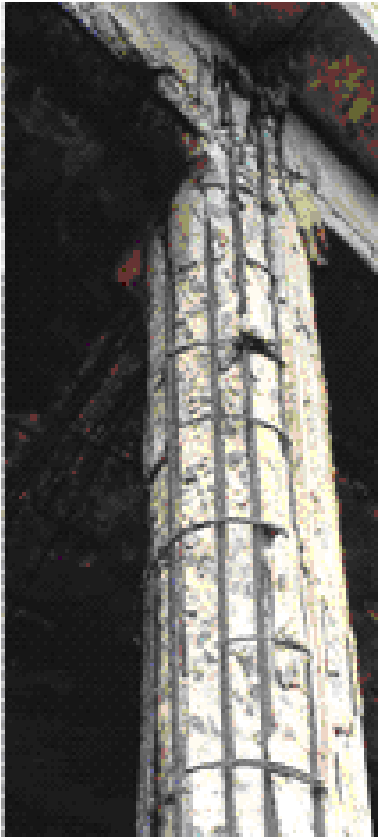
Figure 9.10: Spalling of columns
