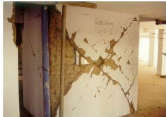
Figure 4.48: RC elevator cores saved many buildings with open ground stories from collapsing. These stiff elements drew large seismic shears and sustained severe cracking
