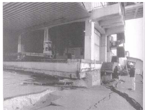
Figure 4.14: Settlement caused by lateral retaining wall movement during the Kobe earthquake. The industrial building is supported by a pile foundation.
