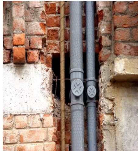
Figure 9.13: Discontinuity of designed structural members
