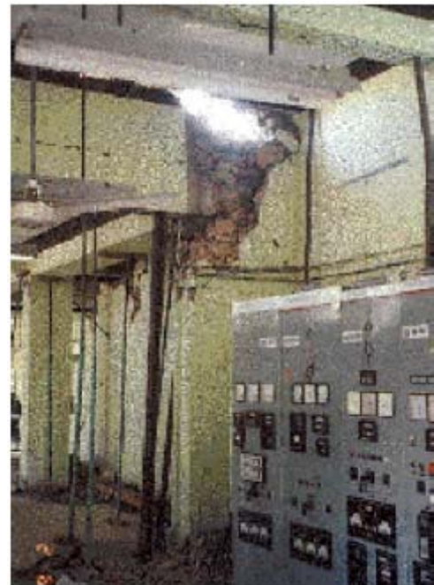
Figure 4.63: Damaged wall inside Anjar substation control building with temporary support column
