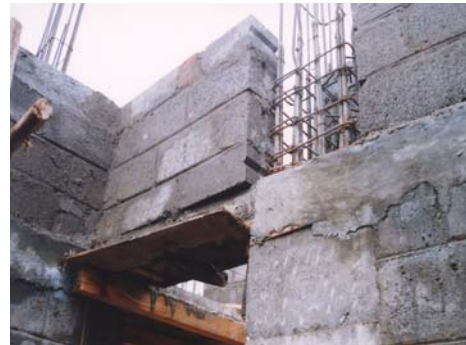
Figure 9.7: Wrong alignment of wall
