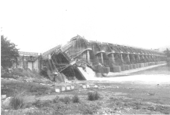
Figure 4.3: Overview of a dam damaged by surface fault rupture associated with the Chi-chi earthquake.
