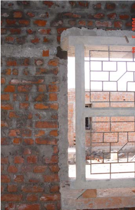
Figure 9.14: Wrong installation of window frame
