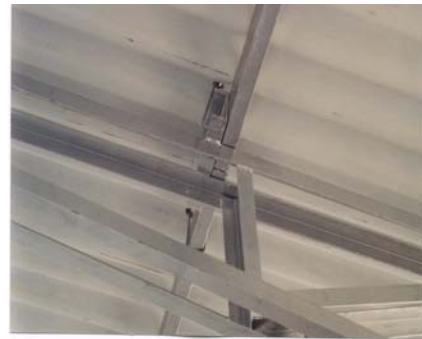
Figure 9.18: Wrong placement of structural members
