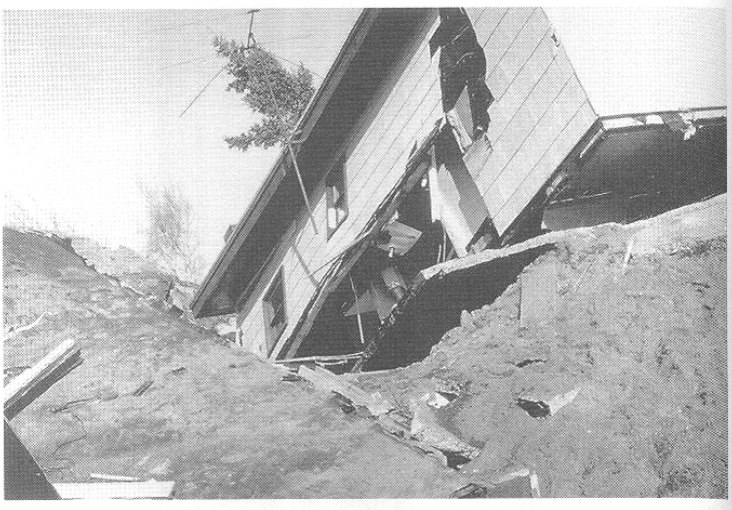
Figure 4.24: Damage caused by movement of the Turnagain Heights landslide during the Alaskan earthquake on March 27, 1964.
