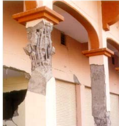
Figure 4.50: Many open ground story buildings did not collapse, but sustained severe damage to the columns in the ground story
