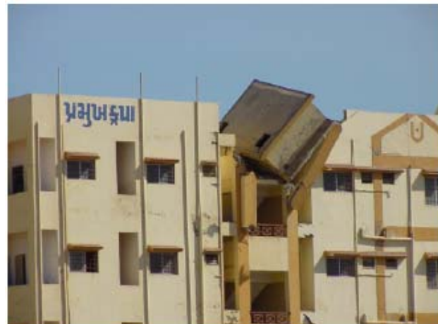
Figure 4.45: Damage to small service water tank on top of RC frame building in Bhuj. Tanks are either nominally or not connected to building frame.
