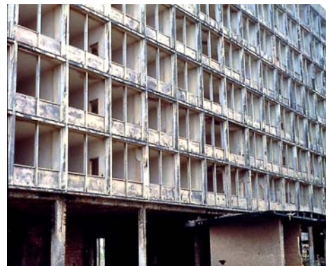
Figure 9.9: Stains and spalling of columns
