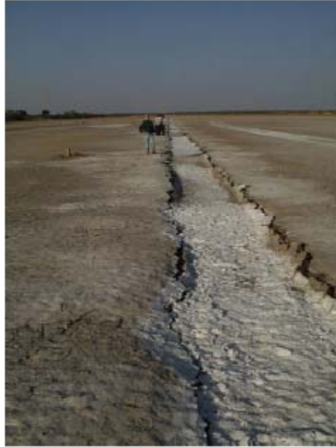
Figure 4.22: Settlement of backfill above natural gas pipeline
