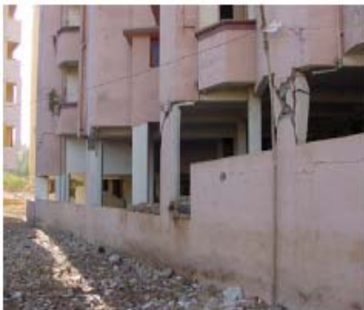
Figure 4.44: damage to perimeter columns of building with varying lateral supports from masonry infills: shear failure in short columns and flexure/shear failure in others.
