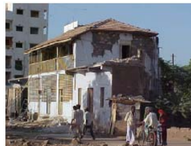
Figure 4.61: Older construction used a large amount of wood in the post and lintel system, thereby providing some lateral resistance to inherently weak stone masonry mud mortar.
