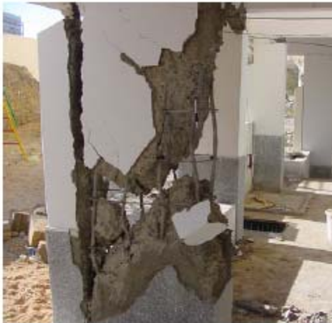
Figure 4.47 Shear cracking of non-ductile columns of an open ground story building in Bhuj
