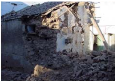
Figure 4.60: Walls built with large stones and no through-stones separated impairing the vertical load carrying capacity.
