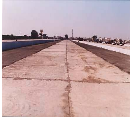
Figure 9.5: Poor road construction
