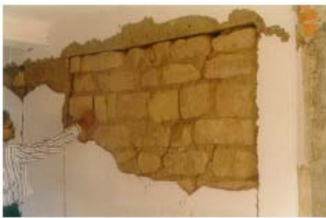
Figure 4.40: Shear cracking in infill masonry in weak cement mortar and sandstone blocks
