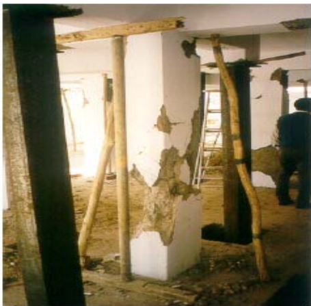
Figure 4.51: Shear failures in columns due to inadequate confinement reinforcement
