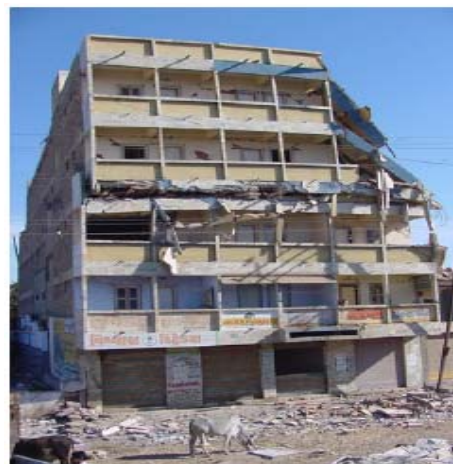
Figure 4.52: Intermediate story collapse in the 6 story building in Bhuj
