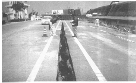
Figure 4.12: Damage on Port Island caused by retaining wall movement during the Kobe earthquake.
