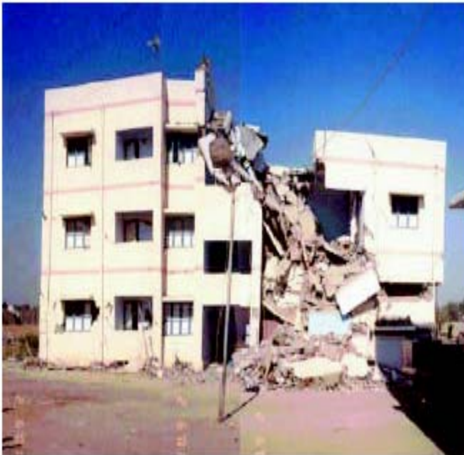
Figure 4.62: Collapsed residential quarters at Anjar substation
