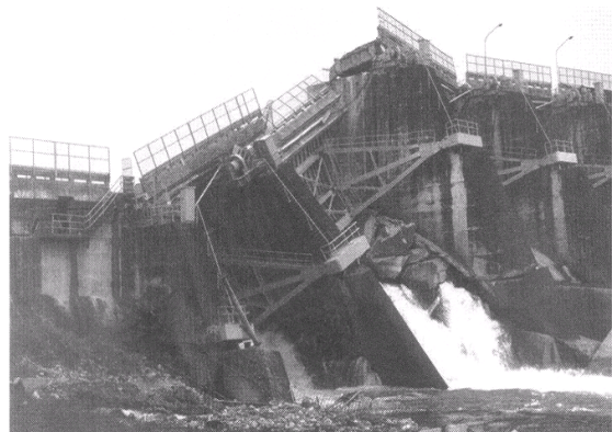
Figure 4.4: Close up view of the location of the dam damaged by surface fault rupture, shown in Fig 4.3
