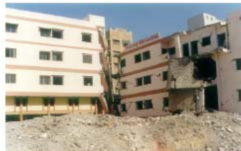
Figure 4.39: Open ground story collapse of short wing of same building
