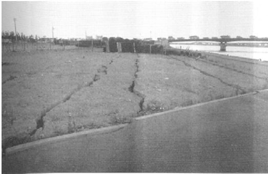
Figure 4.11: Ground cracks caused by lateral retaining wall movement due to liquefaction during the Kobe earthquake. The site is near Nishinomiya Port and consists of reclaimed land.
