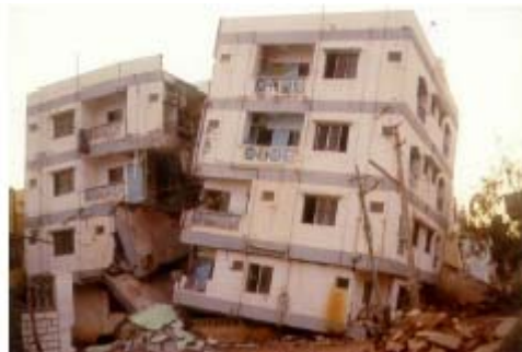
Figure 4.41: Collapse of a partially open ground story building in Bhuj, coupled with vertical split of the building at midline
