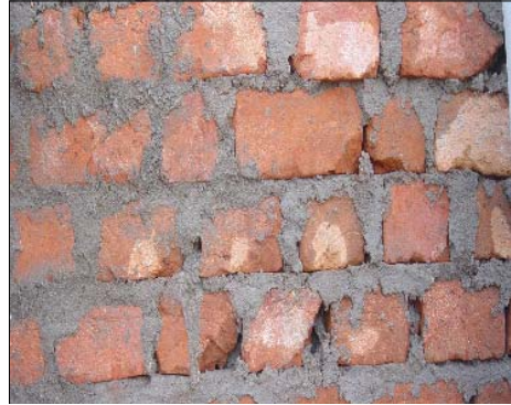
Figure 9.11: Poor workmanship of brick masonry
