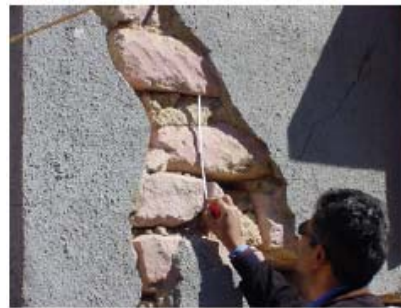
Figure 4.59: Mud mortar is sometimes as thick as 8 cm
