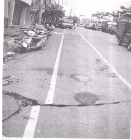
Figure 4.6: Surface fault rupture and roadway damage associated with the Chi-chi earthquake.
