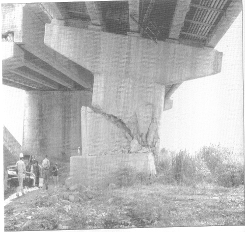
Figure 4.5: Close-up view of bridge pier (Wu-His Bridge) damaged by surface fault rupture-Chi-chi EQ.
