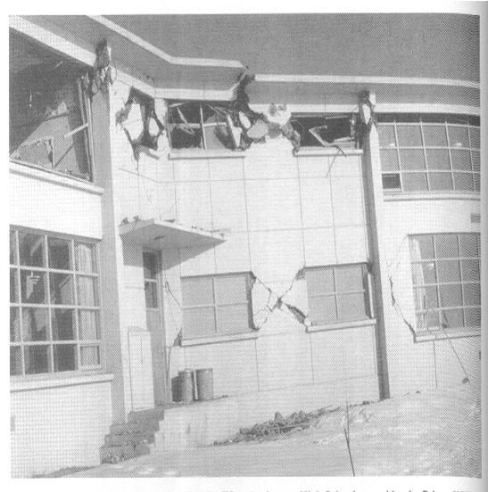
Figure 4.54: Damage to a shear wall at the west Anchorage High School caused by the 1964 Alaskan EQ
