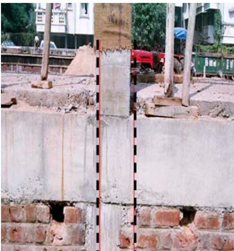
Figure 9.2: Improper alignment of column
