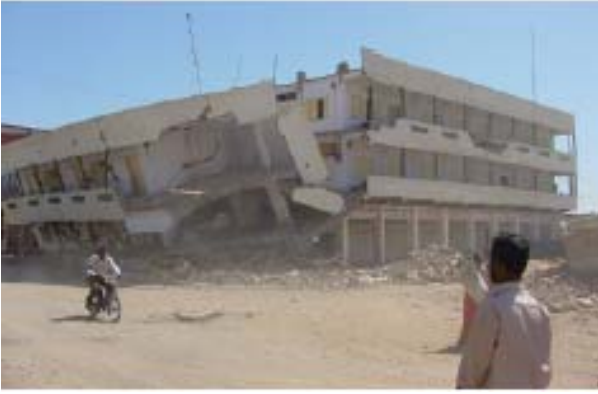
Figure 4.43: Collapse of corner owing to failure of diaphragm at the re-entrant corner of an L-shaped building in Gandhidham
